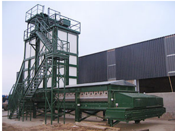
The two chamber VCU system at Gray Composting Services in Aberdeenshire
